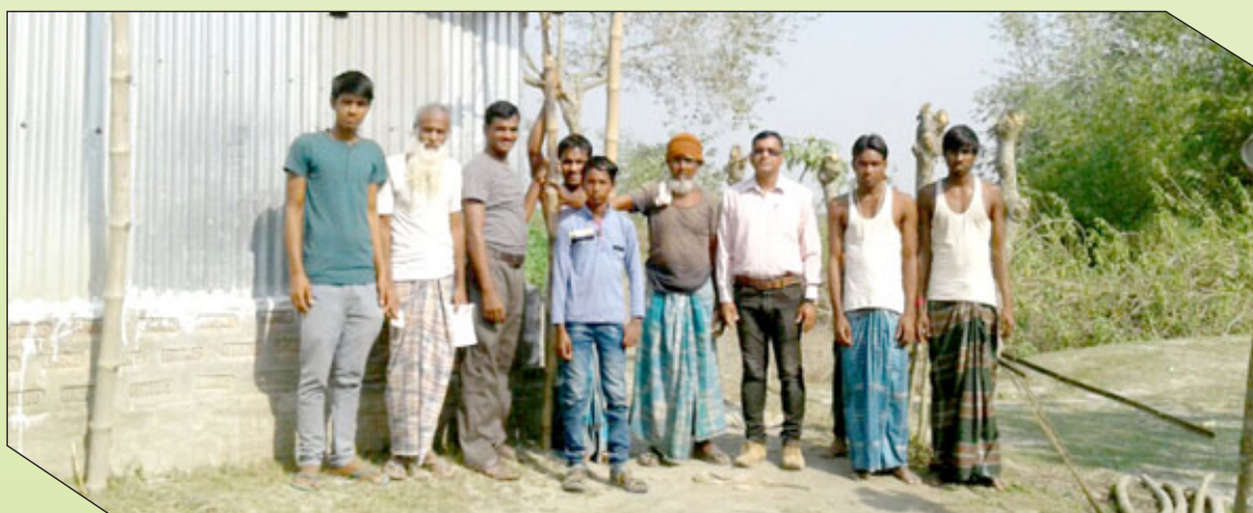
Solar Street Lights being installed at the Airanjongla Pt-II by the Dhubri Unit I Boat Clinic team. Thanks to a philanthropist, remote villages in the Brahmaputra river islands in Assam are being lit up with solar street lights. The donor, Almitra Patel, based at Bengaluru is a member of the Supreme Court committee for Solid waste management for Class 1 cities, Technical expert, Swachh Bharat Mission, Government of India, Clean Jharkhand Project and Ganga ICDP Kanpur
